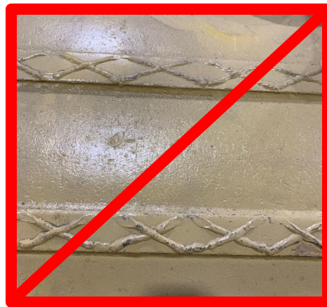
Figure 4 – Incorrect pattern on wear bars
